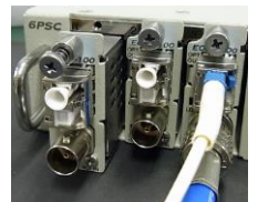
Figure.1 EO converter installation
