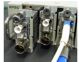
Figure.1 EO converter installation
